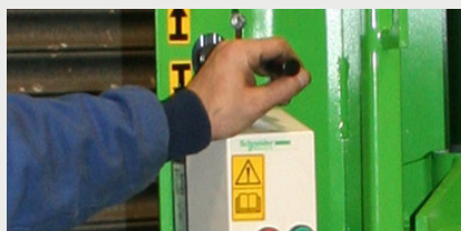
Low-voltage user controls and emergency stop for safe operation
